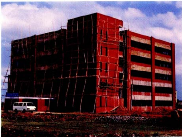
Multistoried Office Building of Bangladesh Institute of Development Science ( BIDS) at Dhaka
